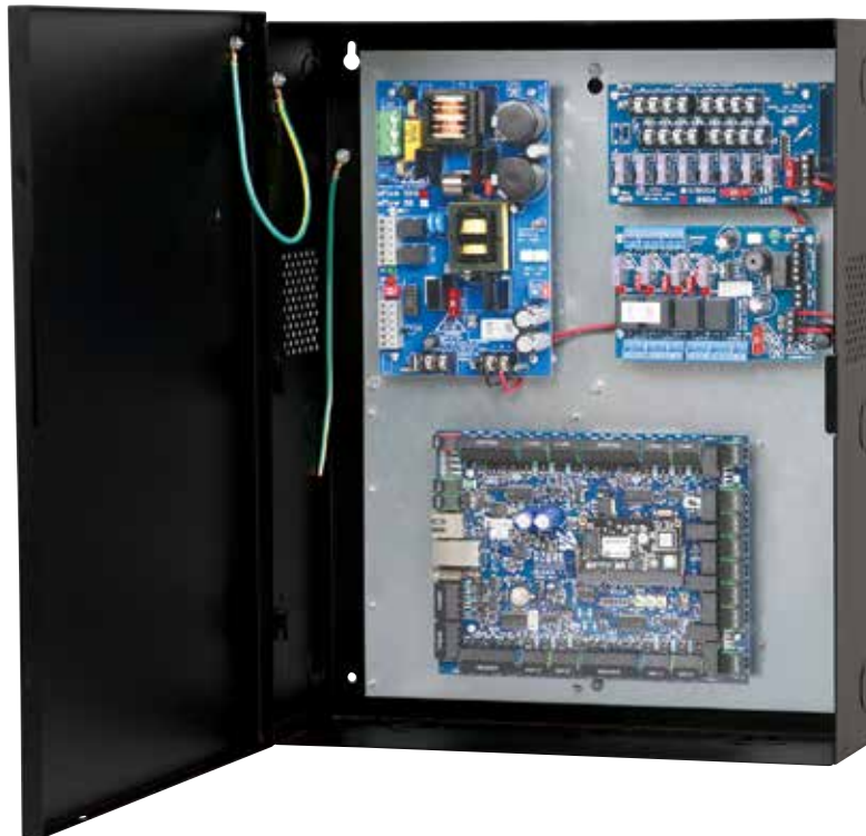
T1AAK3F4S 8-Door Access System with Power
